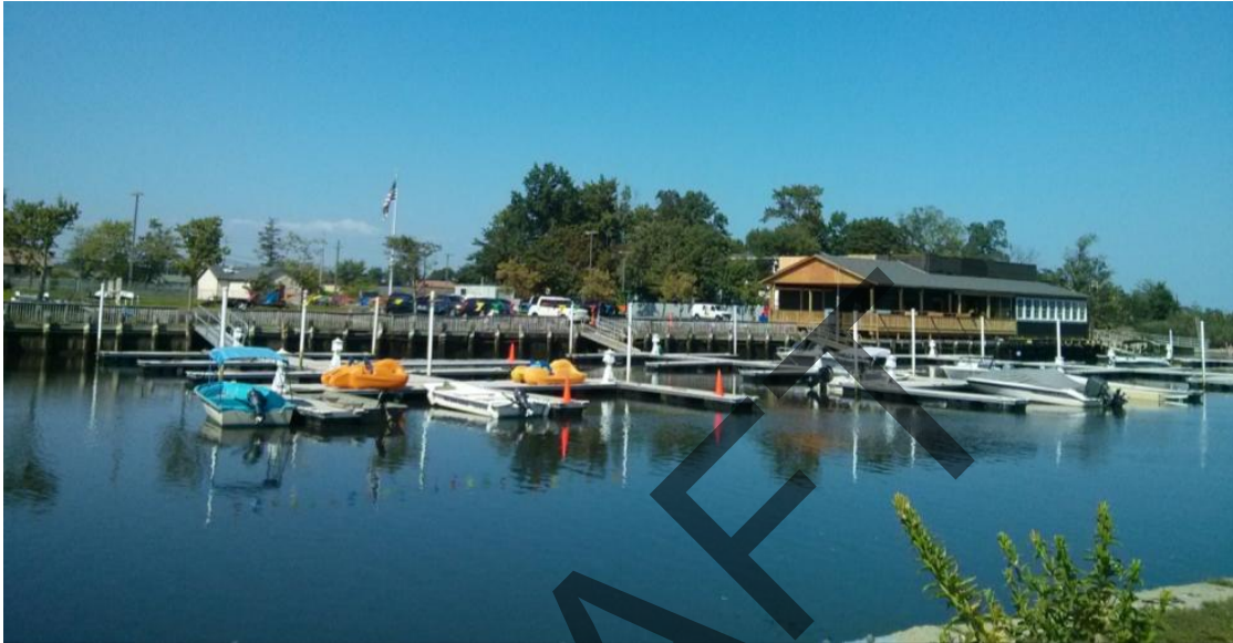
Fort Monmouth Marina in Oceanport, under construction while in operation in August 2014
