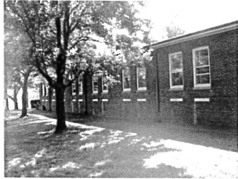
Side addition, note vent infill panels and damaged brick below
